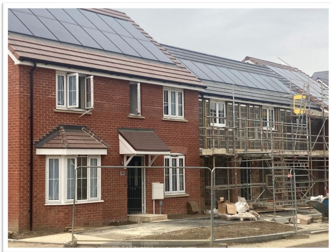
New build with roof solar panels
